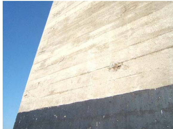
Figure 45. Concrete spall on northwest corner tower, Hangar 2 (Hangar 3 similar).
