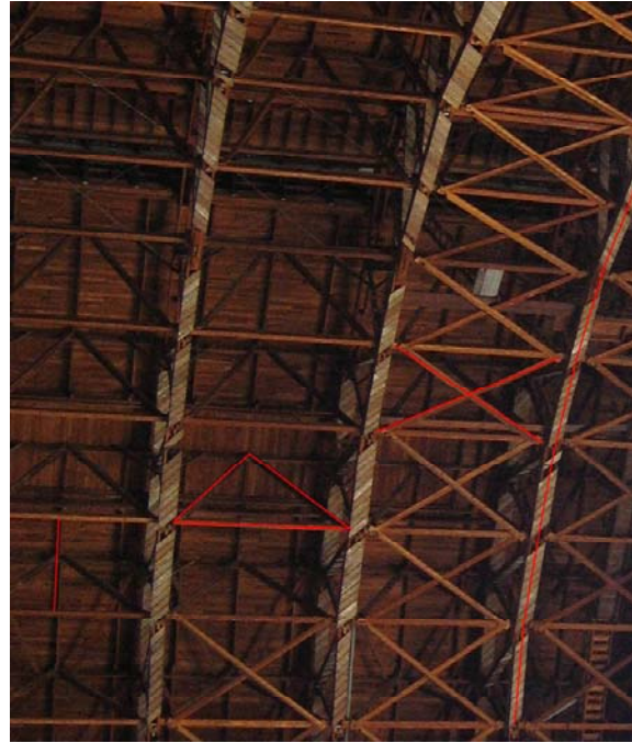
Figure 50. Detail of Structure showing in red, from left to right, purlin, chevron-bracing, X-bracing, and bottom chord of truss. Typical of Hangar 2 and 3.
