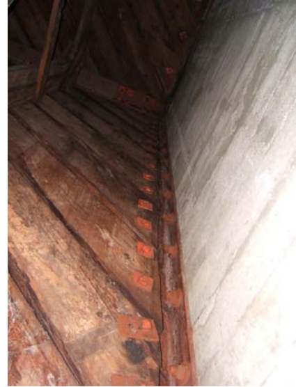
Figure 39. Angle iron union of box girder and corner tower, northeast corner interior corner Hangar 2 (Hangar 3 similar).
