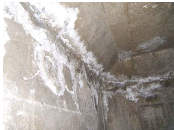
Figure 43 Efflorescence on the interior of the door tower, Hangar 2 southeast tower (Hangar 3 similar).
