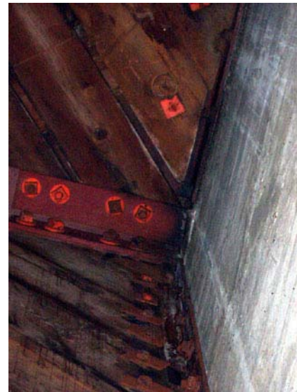
Figure 40. Detail of angle iron at juncture between box girder and corner tower, northeast interior corner Hangar 2 (Hangar 3 similar).
