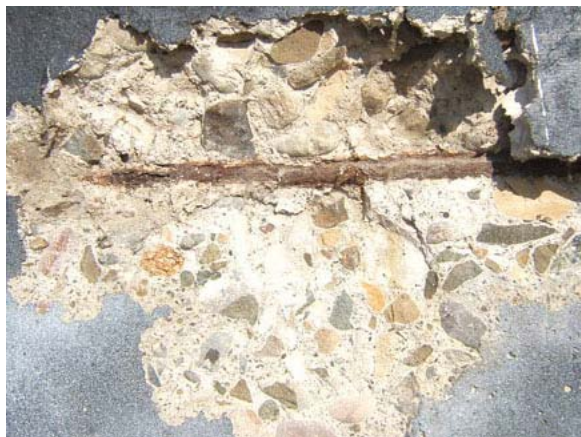
Figure 46. Detail of concrete spall, northwest door tower, Hangar 2 (Hangar 3 similar).
