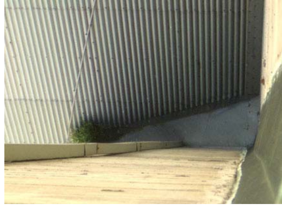
Figure 44 Organic growth found at junction between roof slope and hangar door, Hangar 2 southwest tower (Hangar 3 similar).
