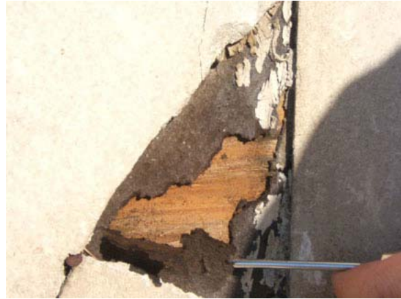
Figure 48. Deteriorated cement asbestos panel showing underlayment of tarpaper and wood substrate, northern corner of the west facade, Hangar 2 (Hangar 3 similar).
