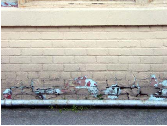
Figure 49. Water table, line of rising damp evaporation causing paint to fail, west façade Hangar 3.
