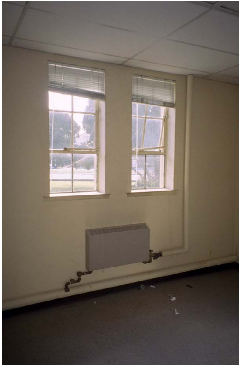
Typical Radiator, Building 24 December 13, 2001
