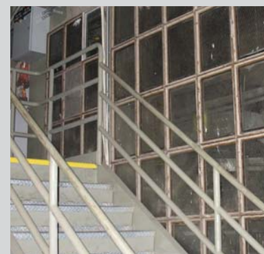
Illustration 6. Multi-lite metal windows and steel stairs on interior are significant features. (Source: ARG, October 2006)
