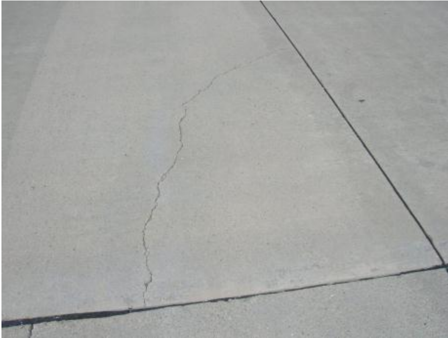
Photo 15. Taxiway B, Section T21C, Low Severity Corner Break.
