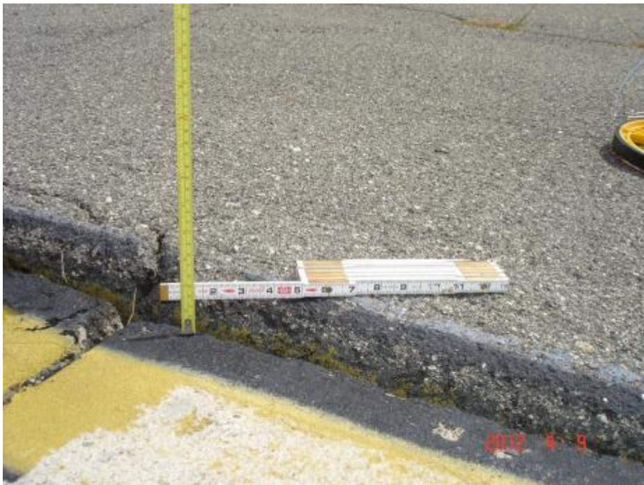
Photo 13. Runway 32L, Section R11A, wide joint between AC and PCC.
