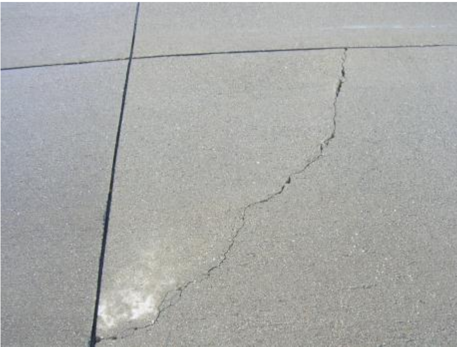
Photo 16. Taxiway A, Section T20C, Medium Severity Corner Break.
