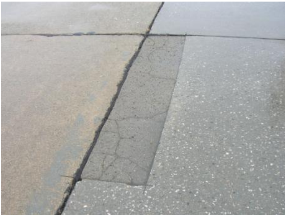
Photo 10. West Apron, Section A22B, Medium Severity Large Patch.
