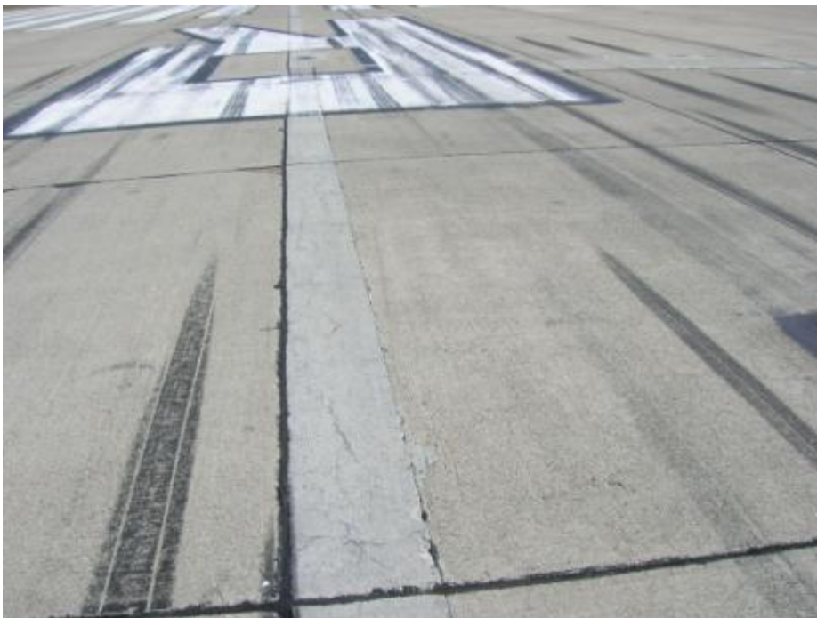
Photo 8. Runway 14L, Section R04A, Medium Severity Large Patch
