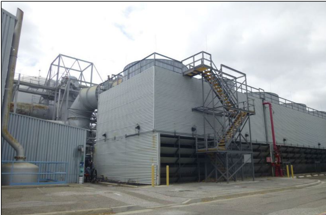
Photograph 14. Cooling towers east of SWS, view to northwest.
