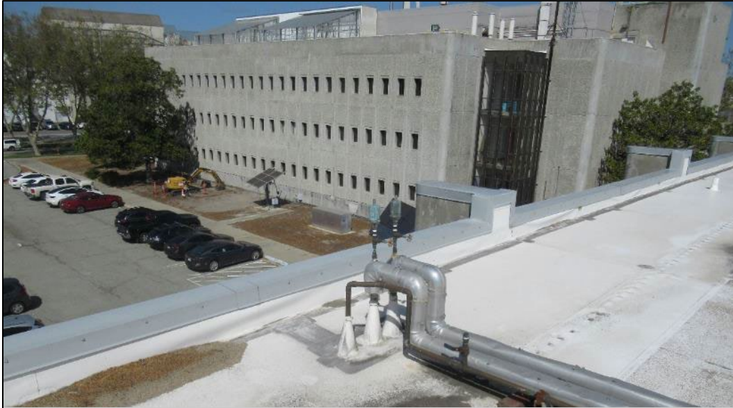
Photograph 17. South and east sides of Building N239 taken from roof of building N239A, view facing northwest.
