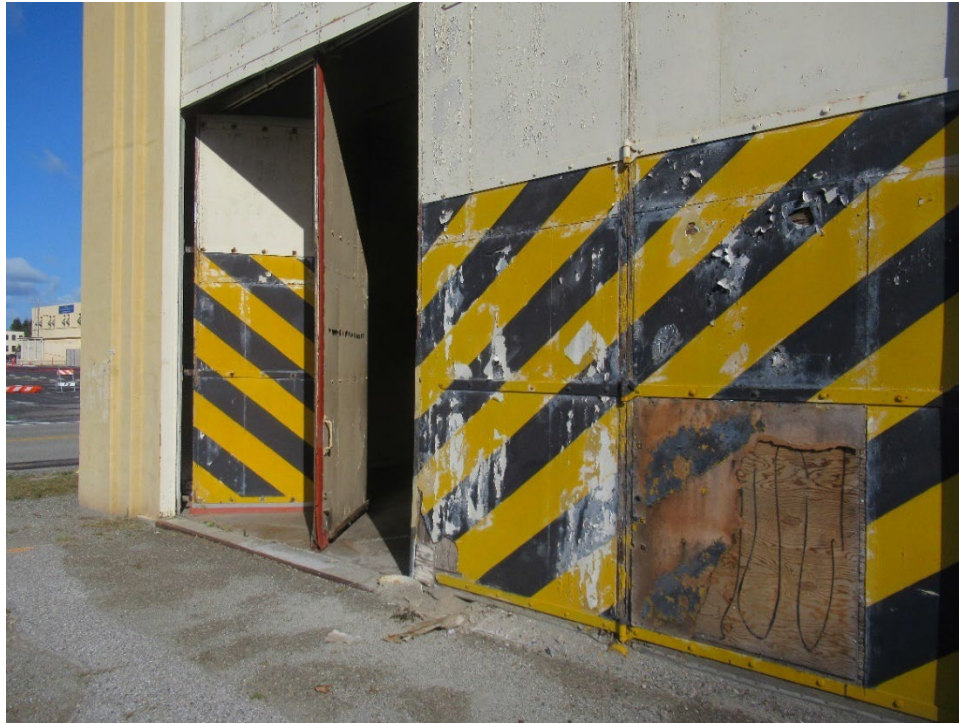
Photograph 3. Detail of deterioration on exterior of bi-fold door and fixed panels on south side of Building 45, view facing northeast.
