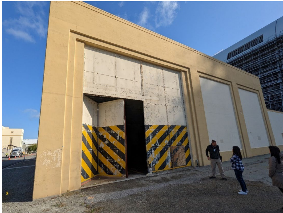
Photograph 2. Exterior view of bi-fold door and fixed panels to be replaced on south side of Building 45, view facing northeast.
