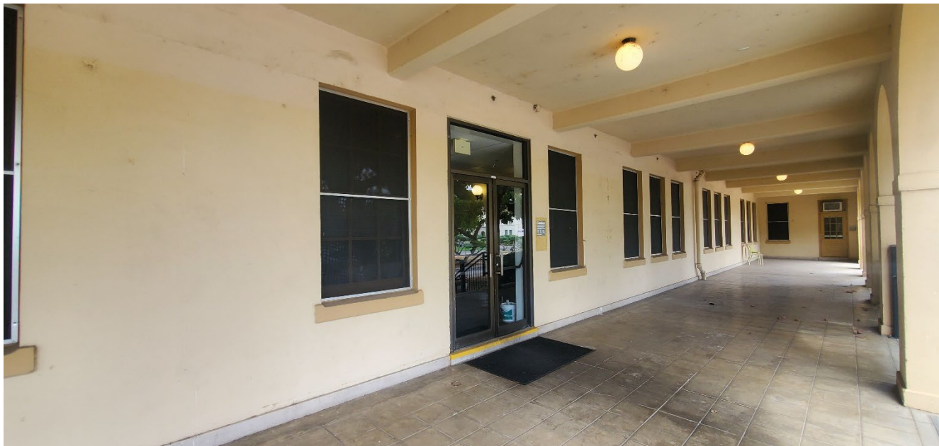
Photograph 5. Building 19 façade (south elevation) showing Conference Room 1218 at east end of arcaded loggia in the first story (far right) inside the eastern projection, view facing east.
