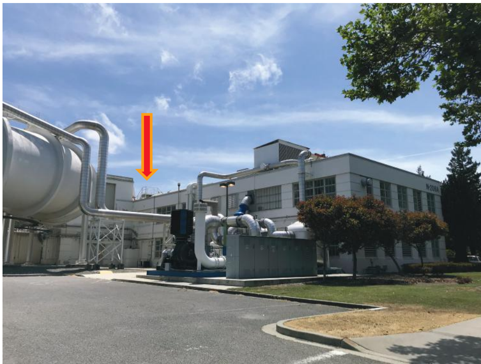
Plate 5. Building N206A, view facing southwest, arrow indicates existing stair to be removed.
