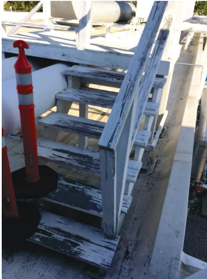
Plate 7. Existing stair to be removed, terminates along the eastern edge of the roof.
