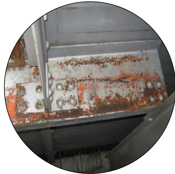
Figure 3-15: Corrosion at Wind Girt Below Window
