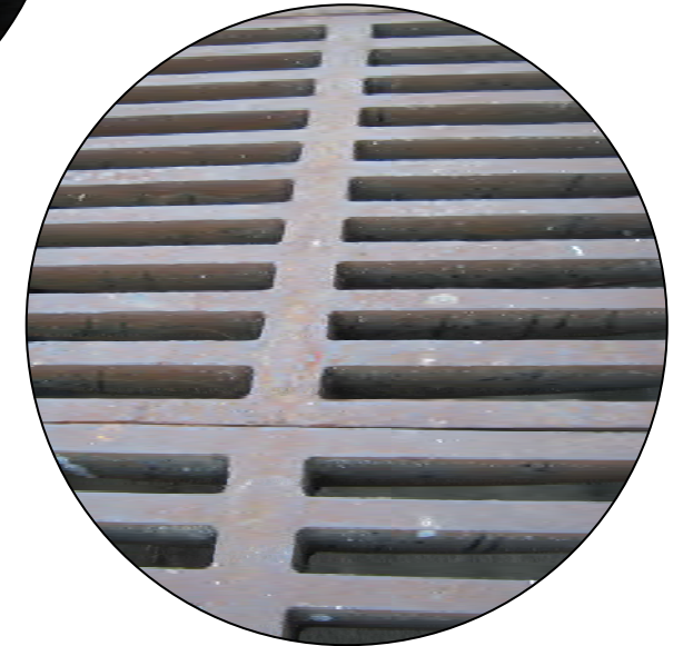
Figure 3-30: Typical Original Grating
