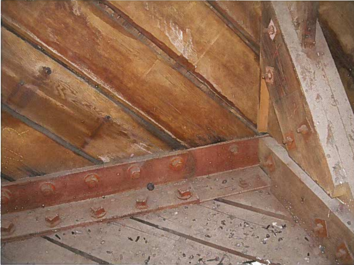
Figure 6. Photograph showing single bolt connections near truss midspan, and double bolt connections at steel angle splice.
