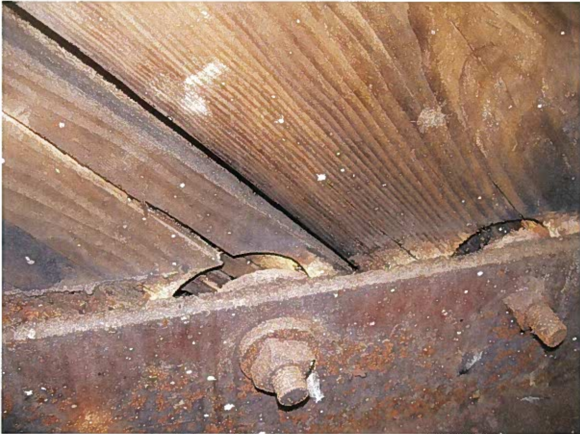
Figure 9. Photograph showing plank to angle connection. Note deformation and splitting of 3x plank members.
