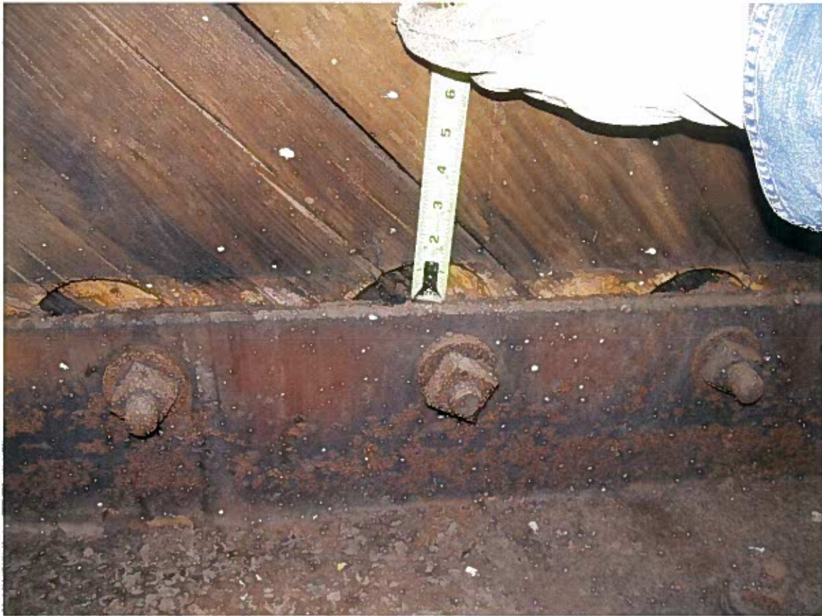
Figure 8. Photograph showing deformation at 3x plank to steel angle connection.
