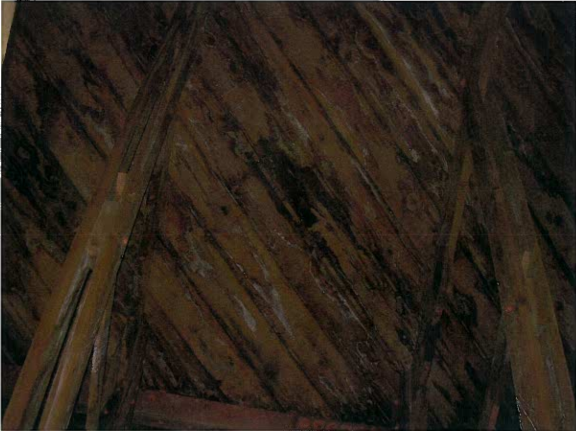
Figure 11. Photograph showing possible water infiltration and damage to truss.
