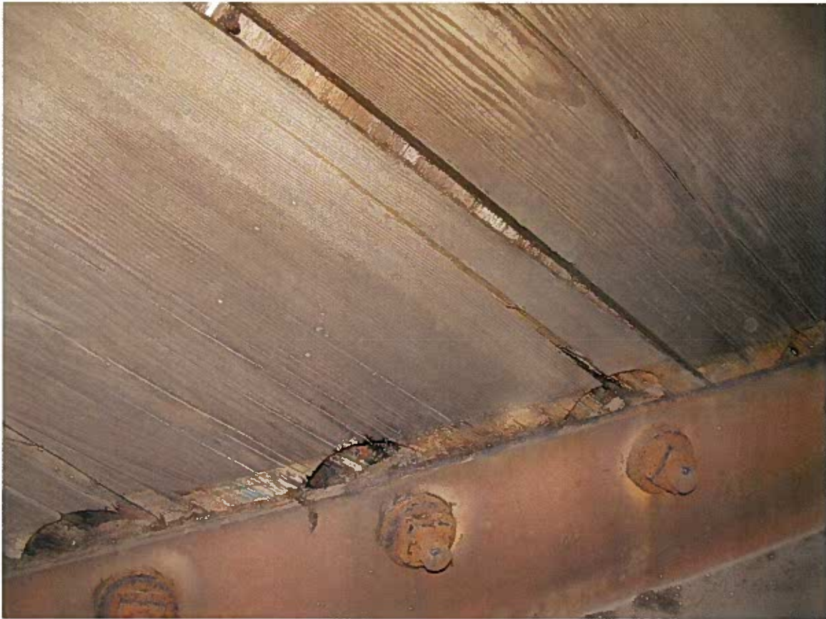
Figure 7. Photograph showing 3x to steel angle connections using two (2) bolts per plank. Note significant deformation at connections and insufficient edge distance.
